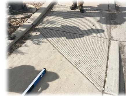
1383469 Curb Ramp No Truncated Domes
