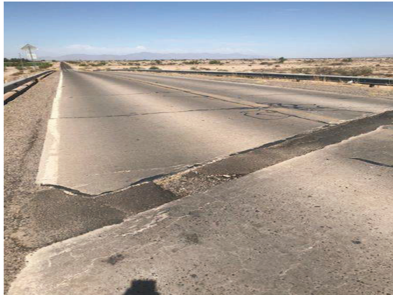
File Name : 01213-2021-05-18-Photo-7.jpg Description : AC deterioration, east approach, with settlement
