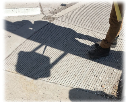
1383464 Curb Ramp No Truncated Domes
