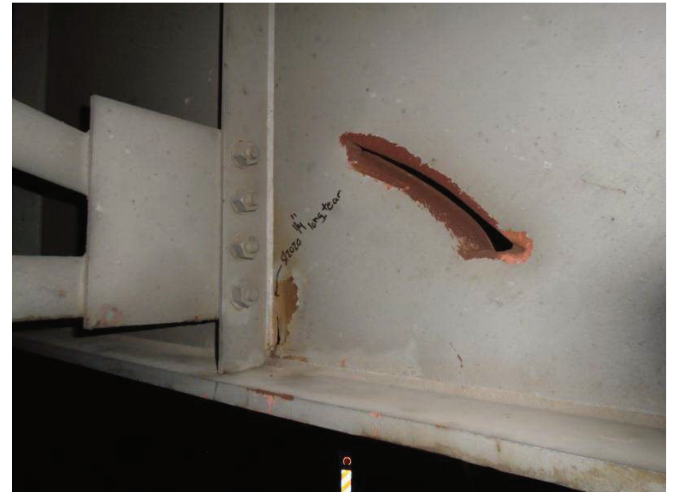
File Name : 01216-2020-05-31-Photo-24.JPG Description : Vertical Tear, Span 2, Girder 2, Diaphragm 1, LN
