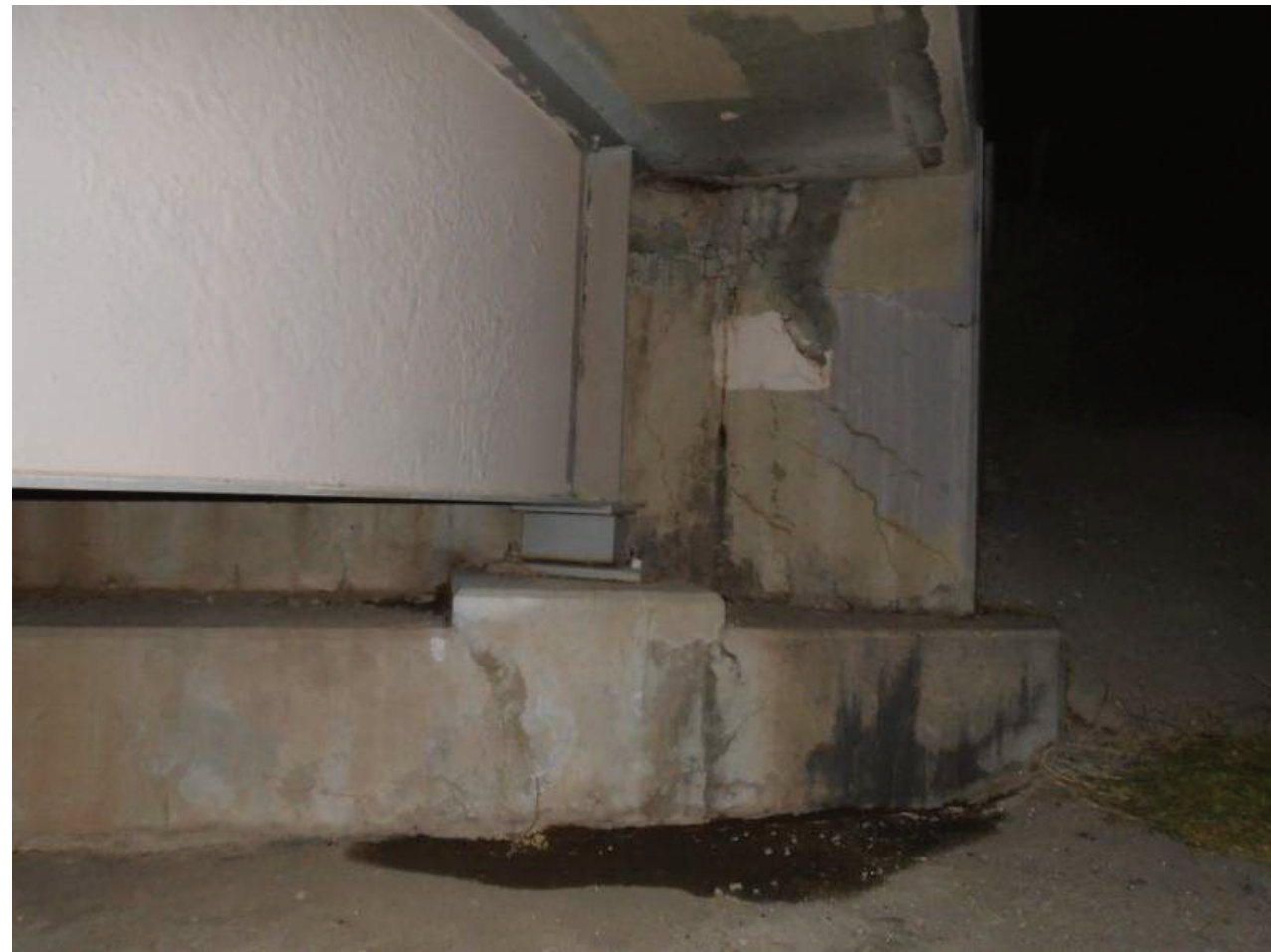
File Name : 01216-2020-05-31-Photo-31.JPG Description : Spalls & Map Cracks, Southwest Abutment Backwall, LW
