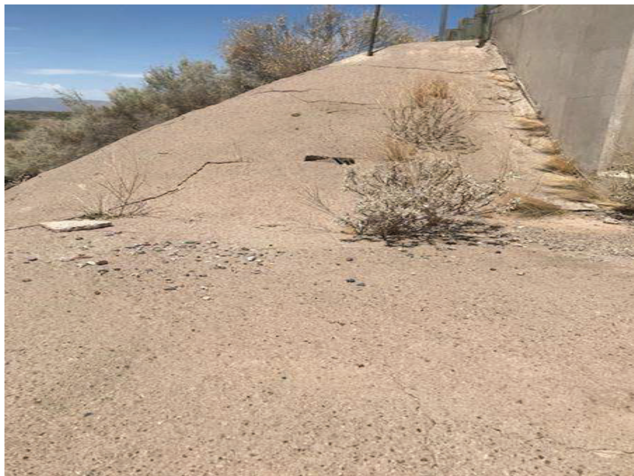
File Name : 01148-2021-05-18-Photo-7.jpg Description : Eroded slope southeast corner
