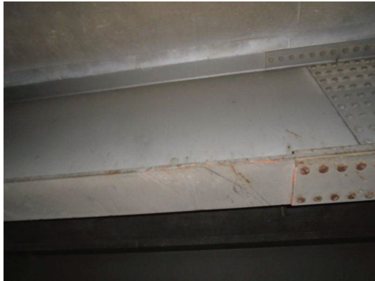
File Name : 01214-2020-05-31-Photo-20.JPG Description : Typical Scrape Marks, Bottom Flange of Girders
