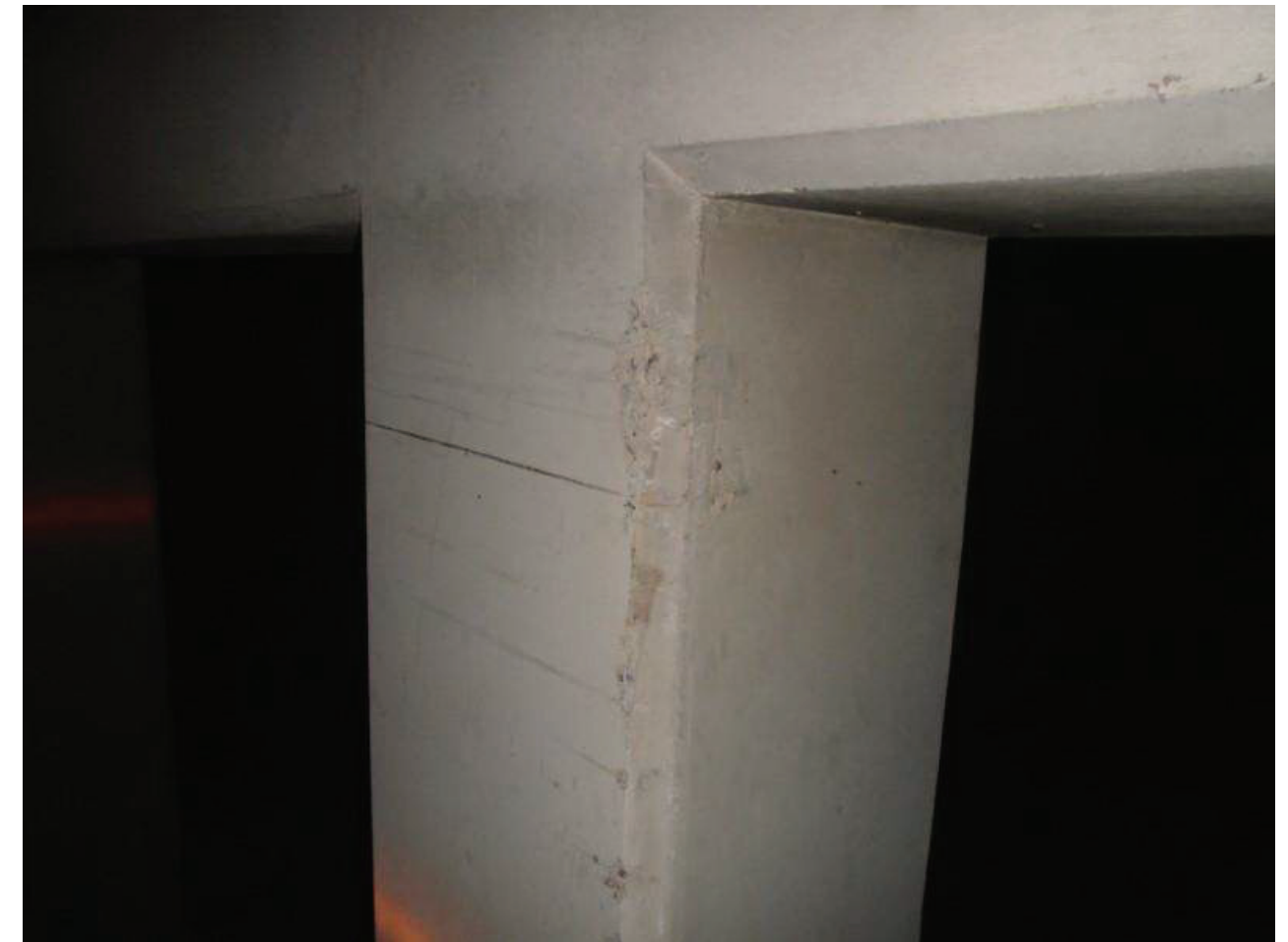
File Name : 01150-2020-05-31-Photo-26.JPG Description : Spall with Scrape Marks, Pier 2, Second Column from East, LE
