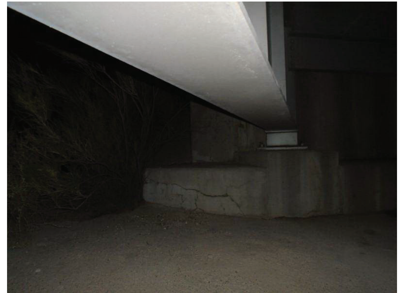
File Name : 01216-2020-05-31-Photo-32.JPG Description : Wide Crack, Northwest Abutment Backwall, LW
