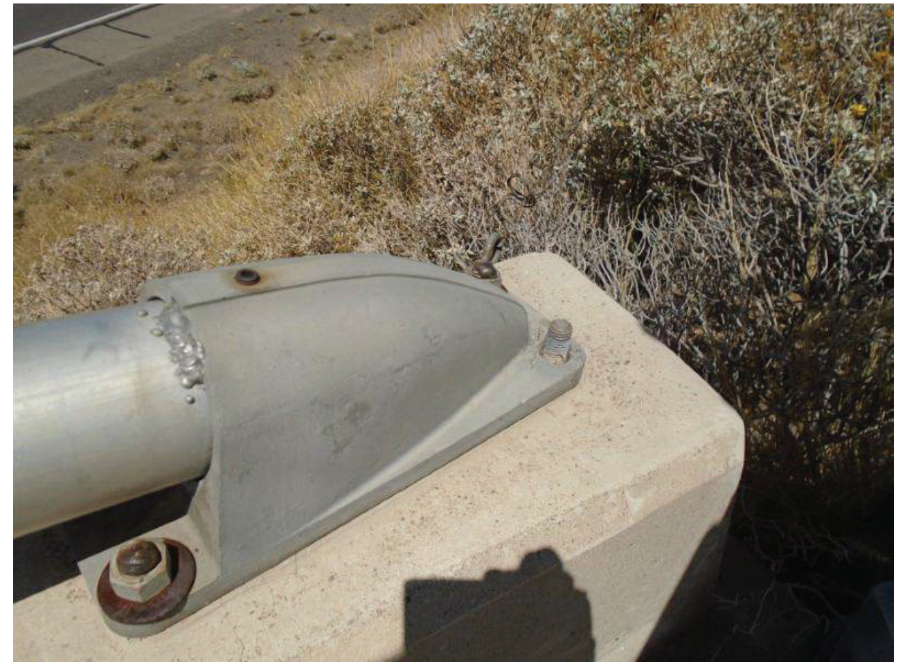
File Name : 01150-2020-05-31-Photo-8.JPG Description : Typical Missing Nuts, End of Metal Railing
