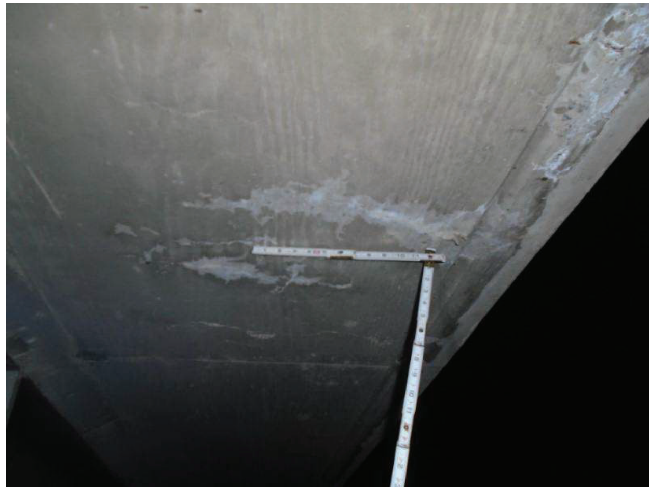
File Name : 01151-2020-05-22-Photo-22.JPG Description : Typical Cracks with Efflorescence, Soffit Overhang
