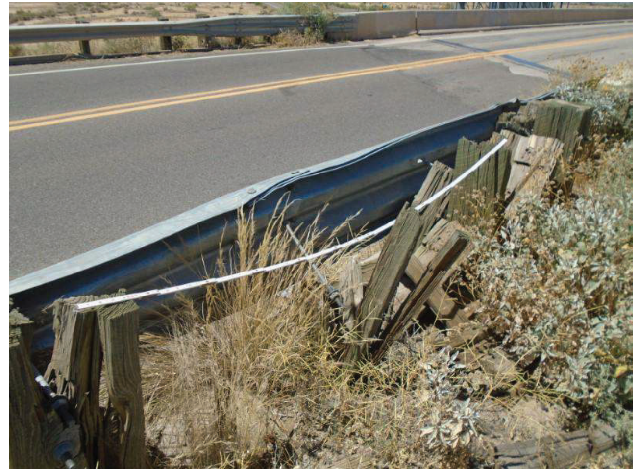
File Name : 01214-2020-05-31-Photo-9.JPG Description : Impact Damage, SE Approach Transition, LN
