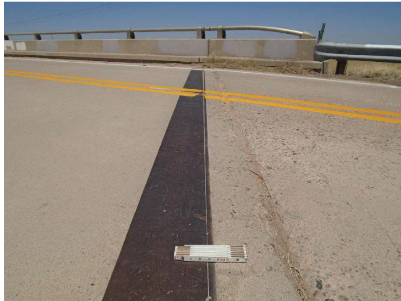
File Name : 01216-2020-05-31-Photo-9.JPG Description : Restricted Joint Movement, East Abutment Joint, LN
