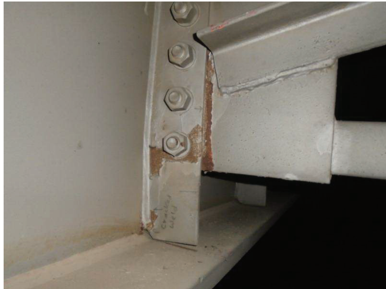
File Name : 01216-2020-05-31-Photo-21.JPG Description : Cracked Weld, Span 2, Girder 1, Diaphragm 1, LSW
