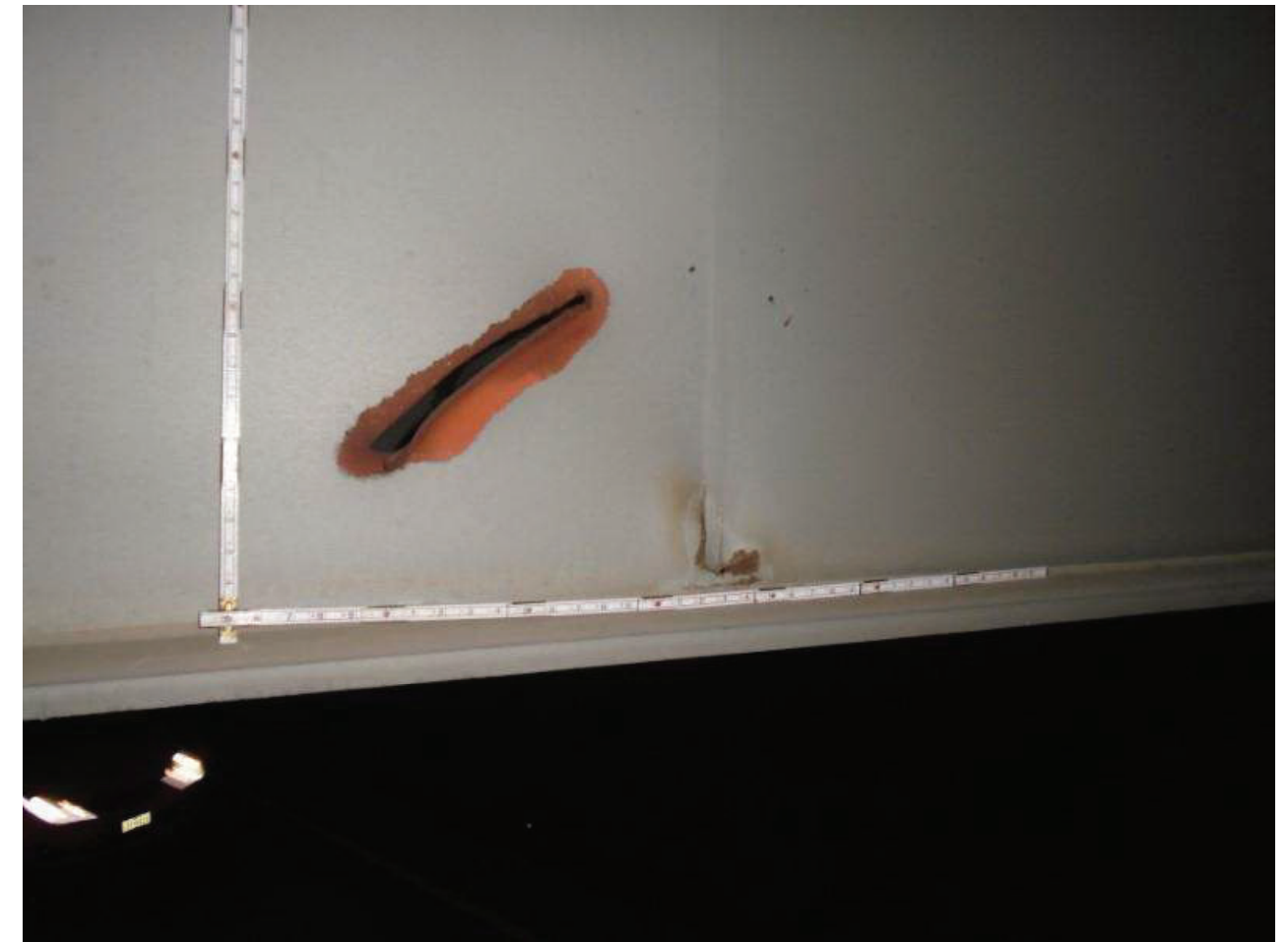
File Name : 01216-2020-05-31-Photo-22.JPG Description : Impact Damage, Span 2, Girder 2, Diaphragm 1, LS
