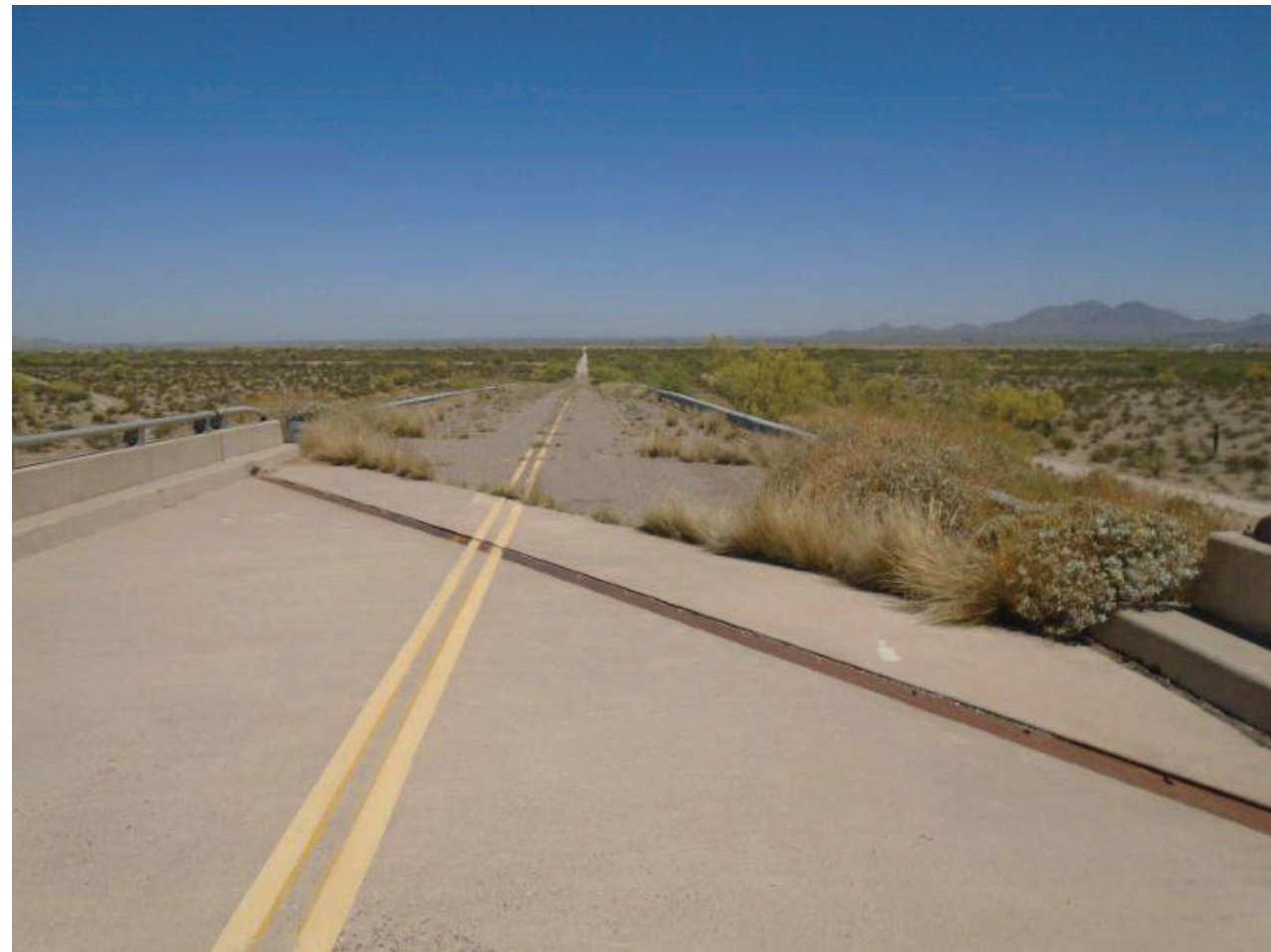
File Name : 01150-2020-05-31-Photo-7.JPG Description : Overgrowing Vegetation, N Approach, LN
