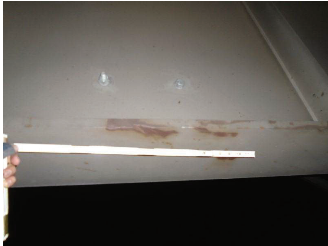
File Name : 01150-2020-05-31-Photo-25.JPG Description : Impact Damage, Span 2, Girder 4, Over Left Lane, LE
