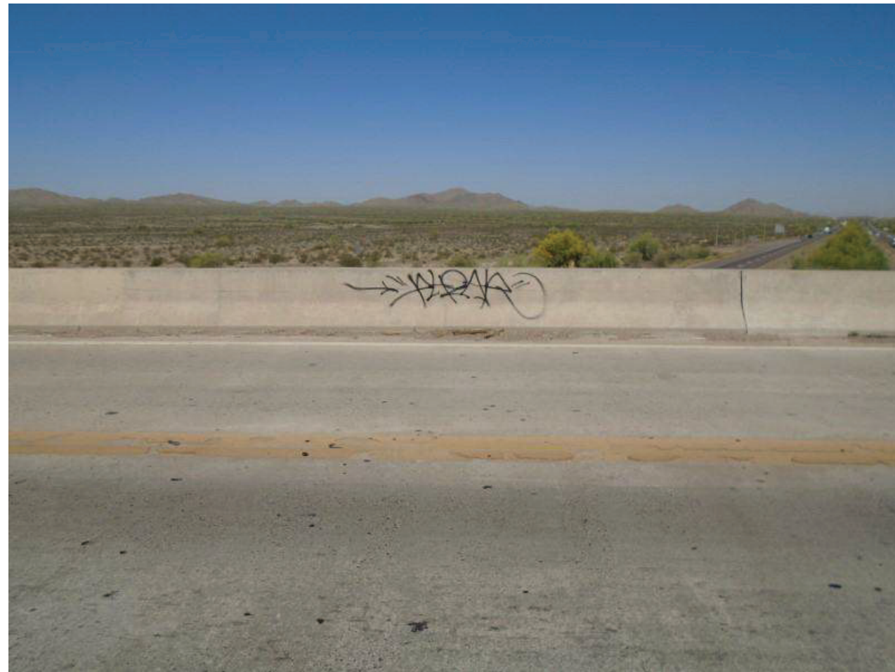
File Name : 01151-2020-05-22-Photo-8.JPG Description : Typical Graffiti, Concrete Bridge Barrier
