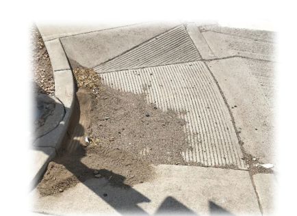
1383476 Curb Ramp Gravel on Ramp
