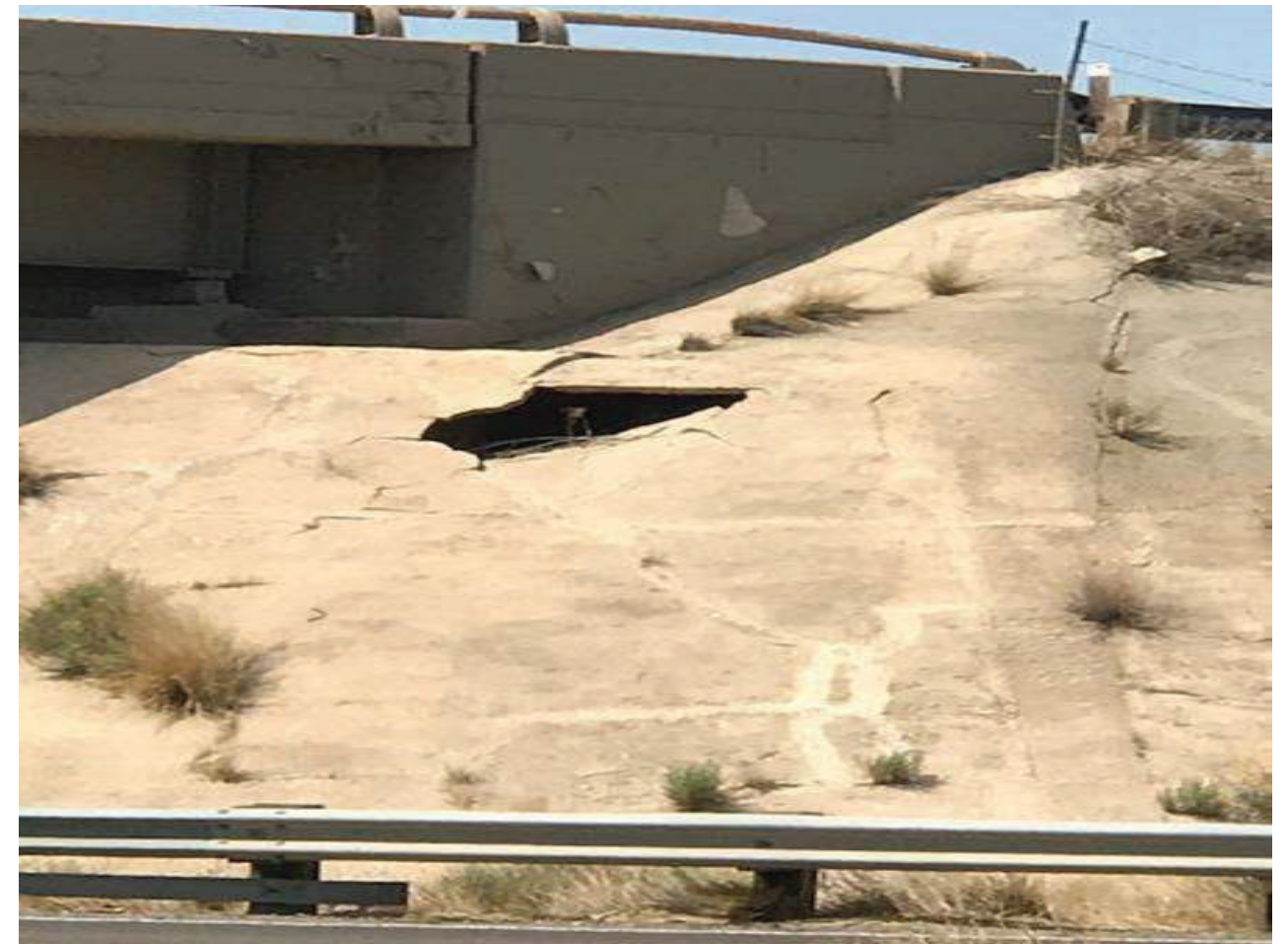
File Name : 01149-2021-05-18-Photo-6.jpg Description : Eroded slope pave at E and W abutments
