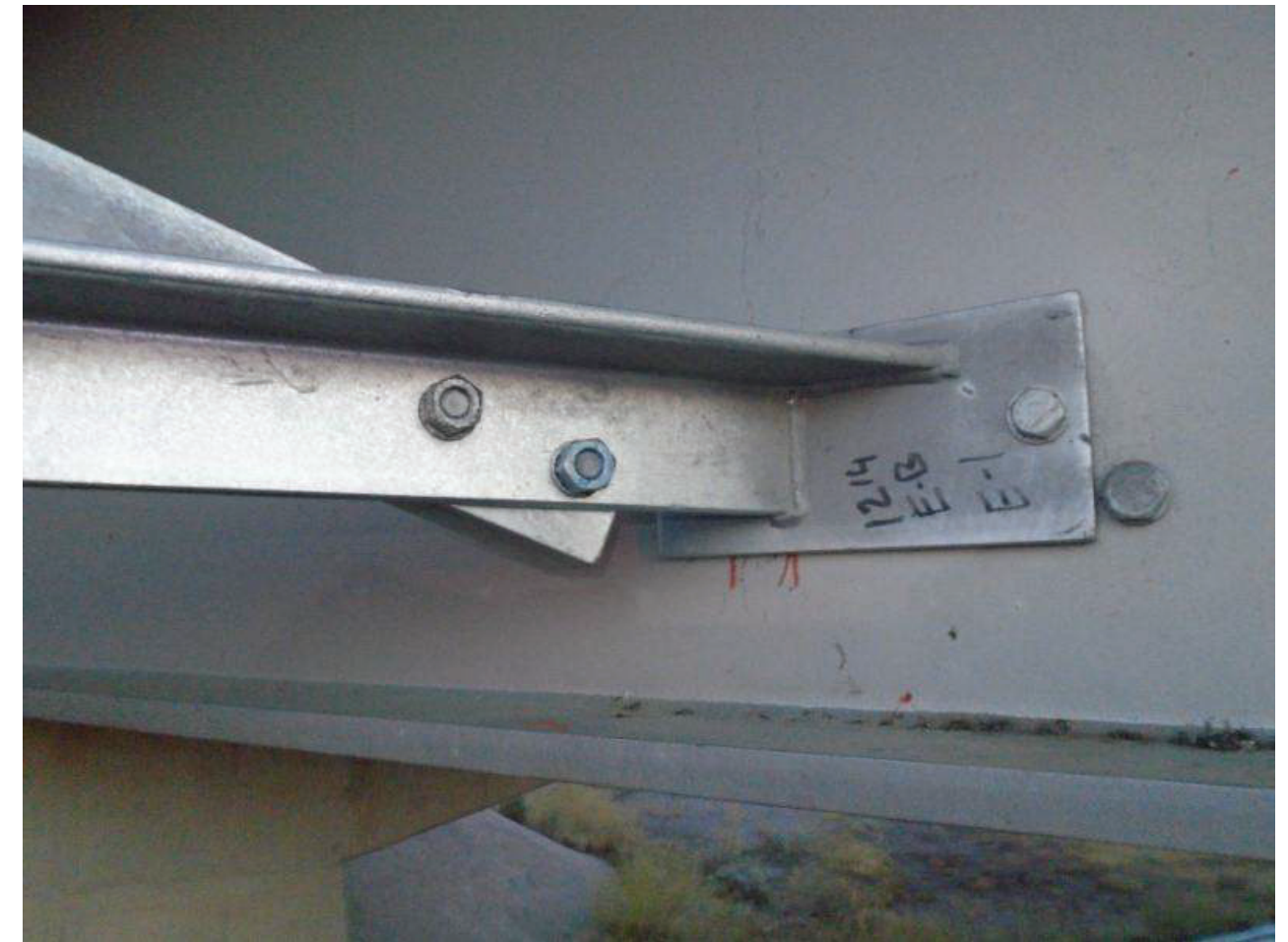
File Name : 01214-2020-05-31-Photo-25.JPG Description : Hand Tight Connection, Wrong Way Sign Support, Span 3, LSW
