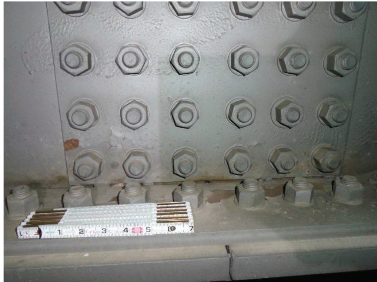
File Name : 01151-2020-05-22-Photo-20.JPG Description : Typical Chipping Paint, Girder 1, Span 2, LW
