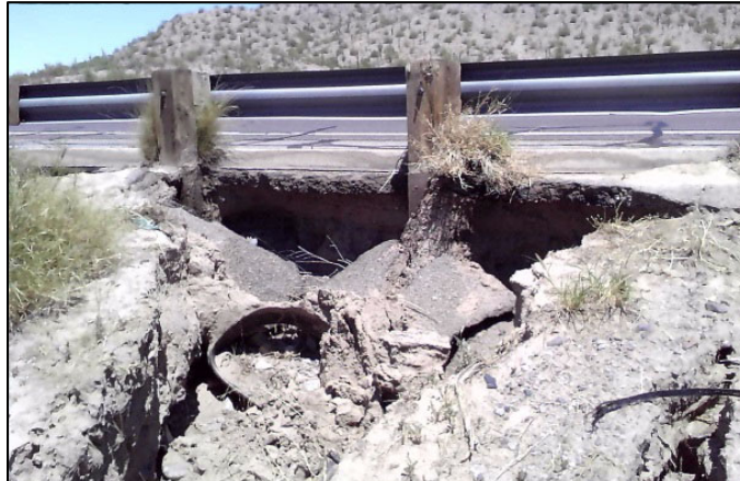
Figure 7: Erosion under Curb and Pavement I-10 EB MP 173.07
