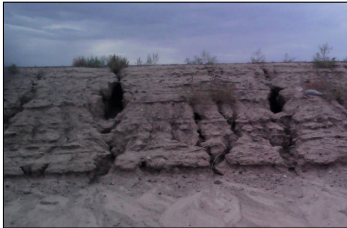
Figure 8: Slope erosion I-10 WB MP 173.14
