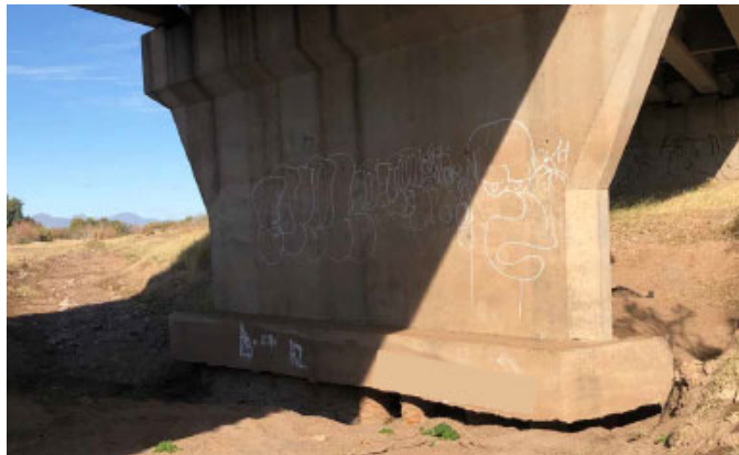
Figure 2: River Erosion Has Exposed Foundations
