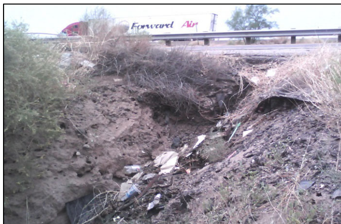
Figure 9: Slope erosion I-10 EB MP 173.13
