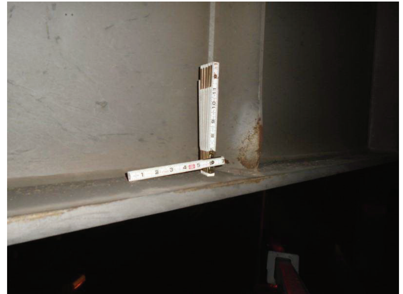
File Name : 01150-2020-05-31-Photo-24.JPG Description : Cracked Diaphragm Stiffener, Span 4, Girder 2, Bay 2, LW
