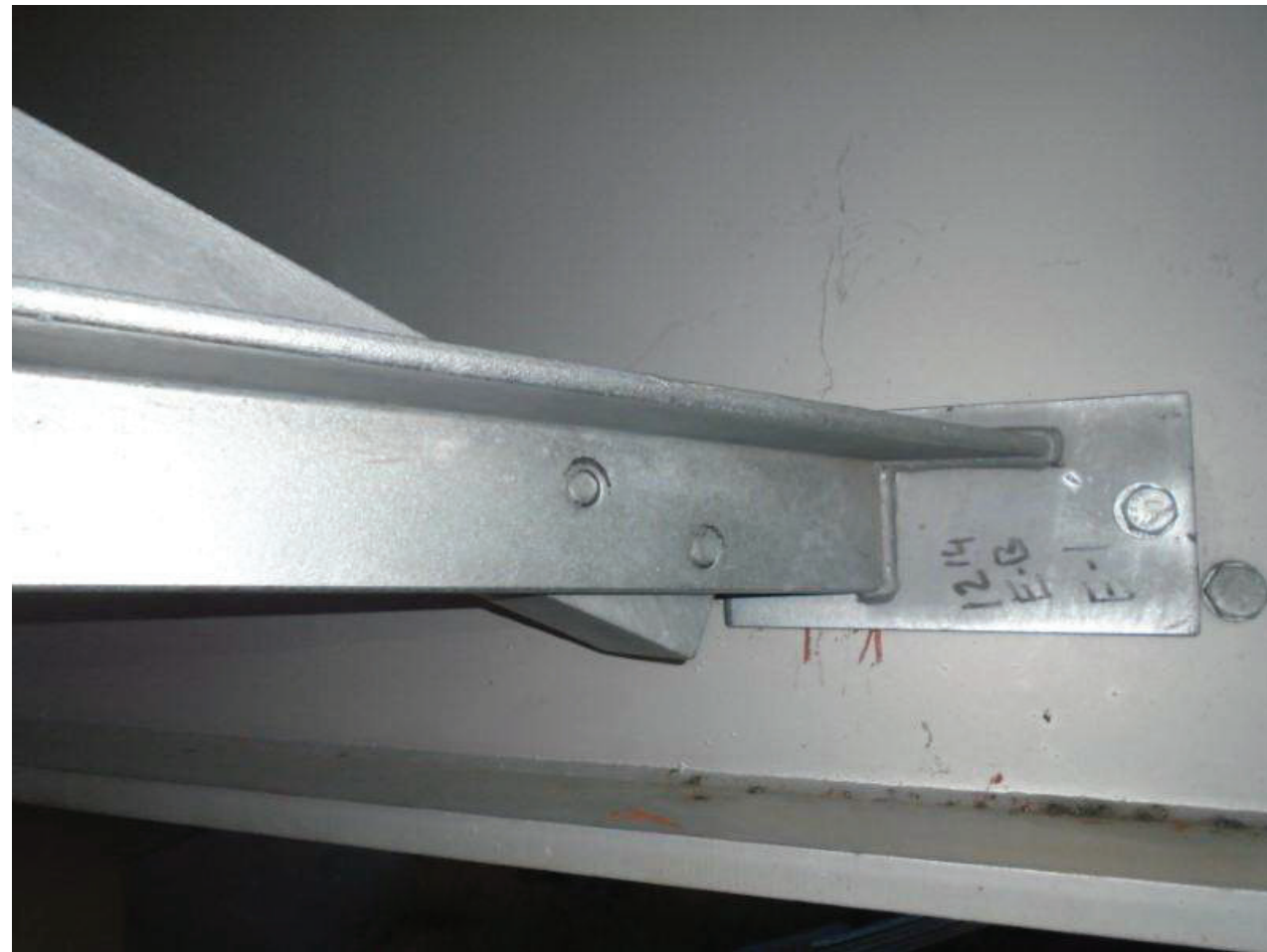
File Name : 01214-2020-05-31-Photo-24.JPG Description : Loose Connection, Wrong Way Sign Support, Span 3, LSW
