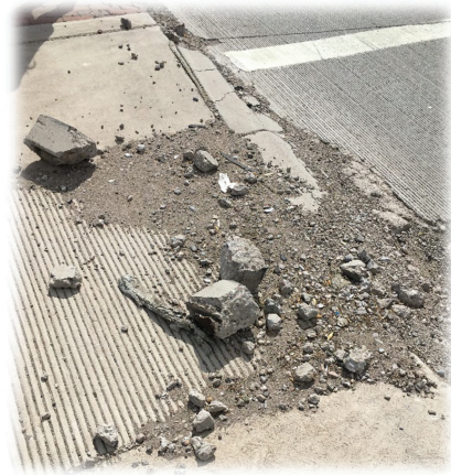
1383470 Traffic Island Cracked Concrete
