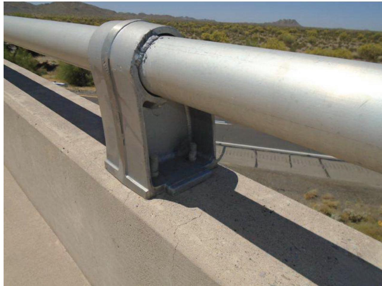
File Name : 01150-2020-05-31-Photo-9.JPG Description : Typical Missing Nuts, Intermediate Metal Railing Support
