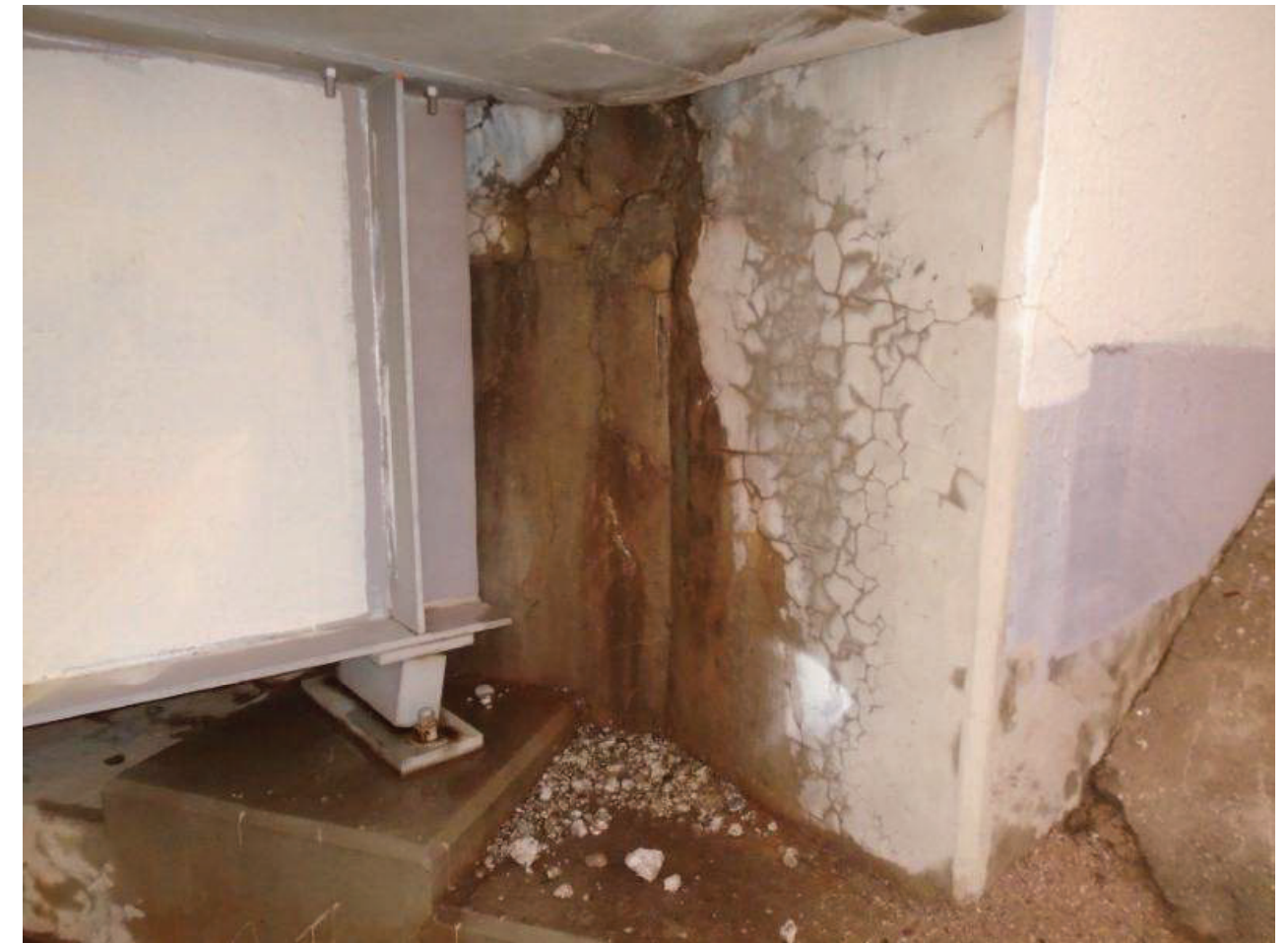
File Name : 01216-2020-05-31-Photo-30.JPG Description : Spalls & Map Cracks, Southeast Abutment Backwall, LNE
