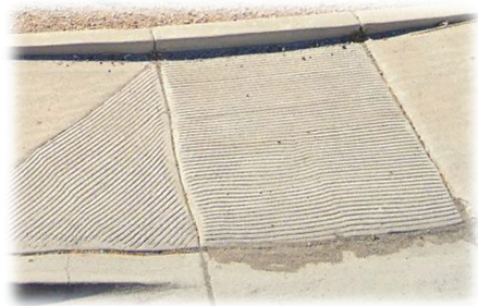
1383479 Curb Ramp No Truncated Domes
