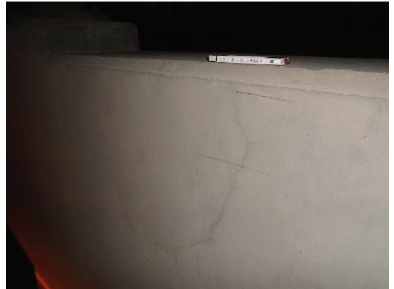
File Name : 01214-2020-05-31-Photo-27.JPG Description : Typical Pier Cap Cracks
