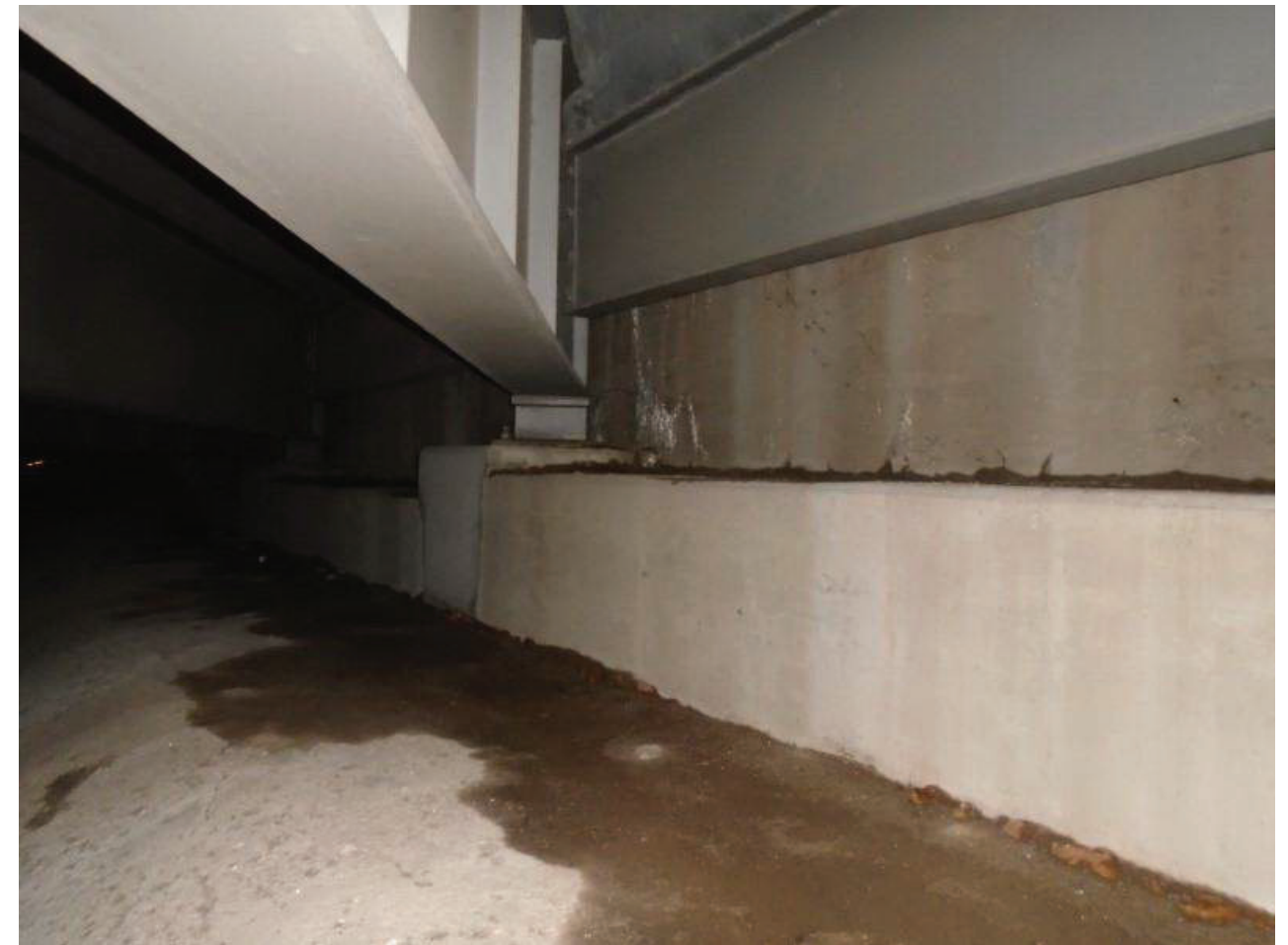
File Name : 01215-2020-05-31-Photo-9.JPG Description : North Abutment, LNW
