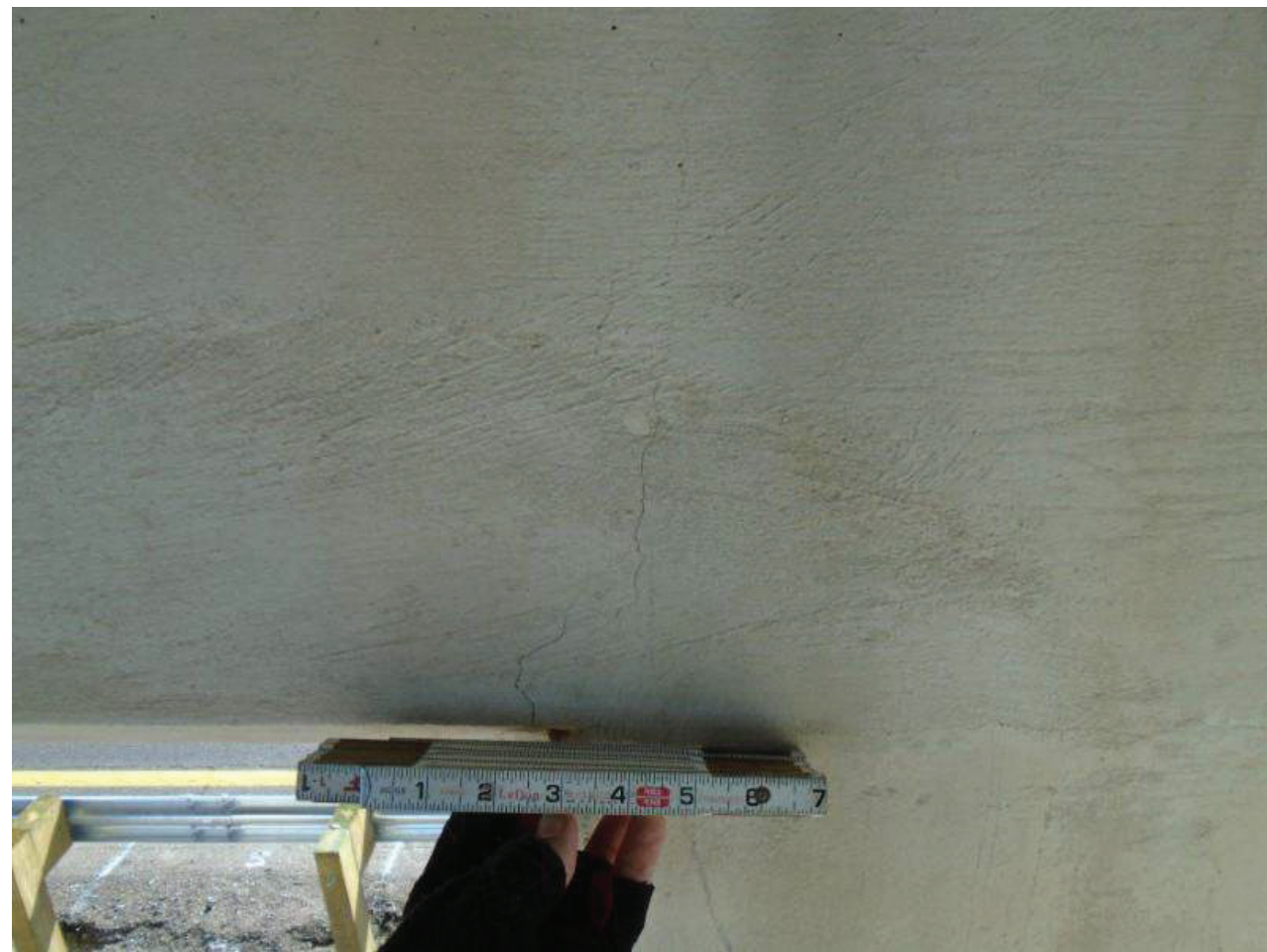
File Name : 01150-2020-05-31-Photo-27.JPG Description : Vertical Cracks, Pier 3 Cap, at Column 4, LN
