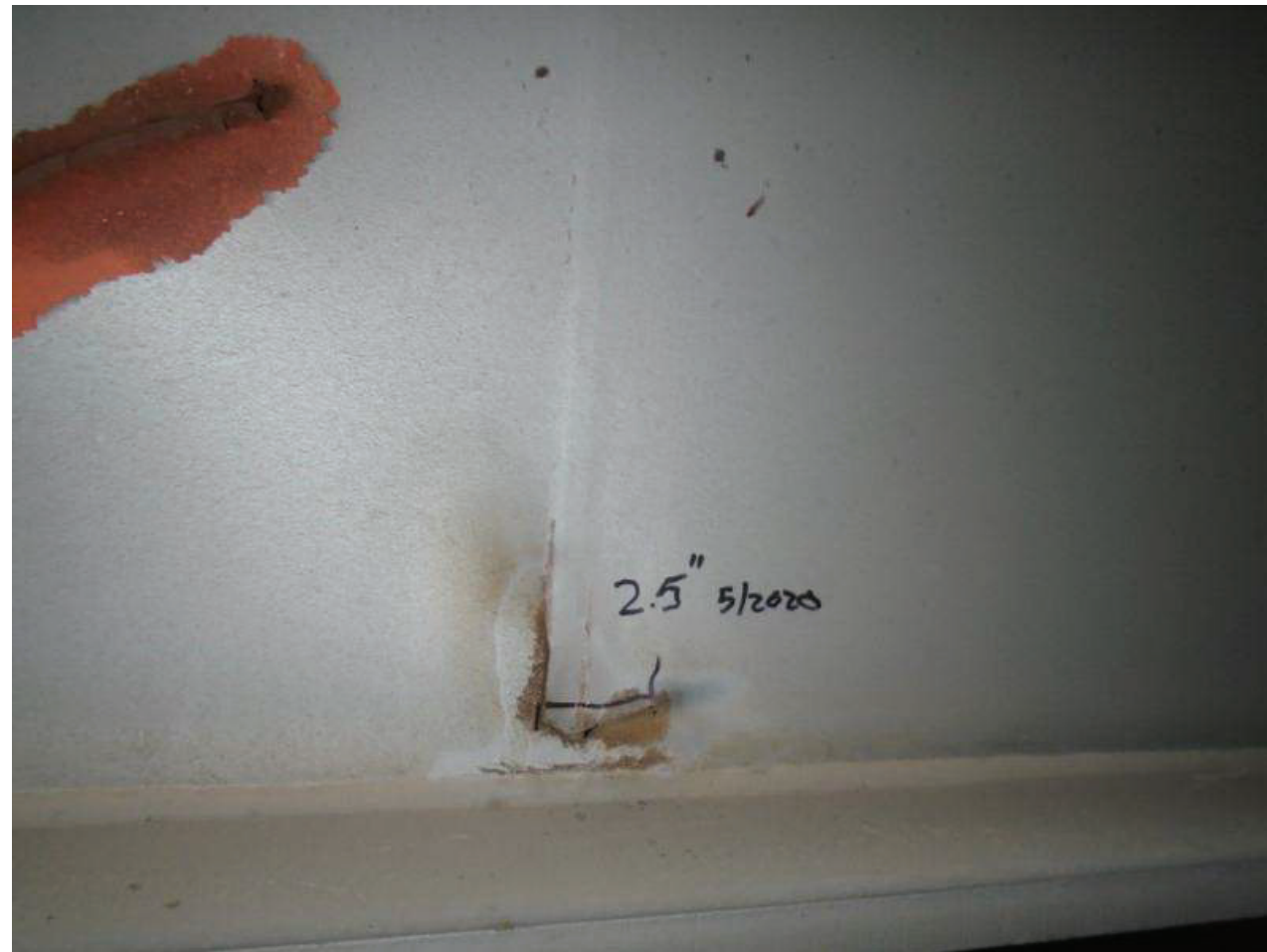
File Name : 01216-2020-05-31-Photo-25.JPG Description : Horizontal Tear/Crack Span 2, Girder 2, Diaphragm 1, LS
