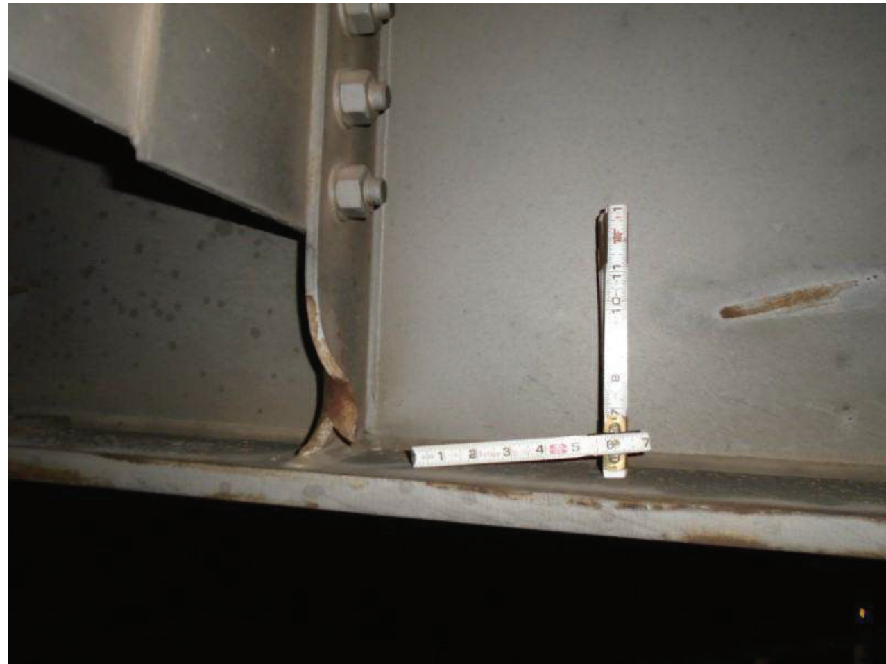
File Name : 01150-2020-05-31-Photo-23.JPG Description : Bent Diaphragm Stiffener, Span 4, Girder 2, Bay 2, LSW
