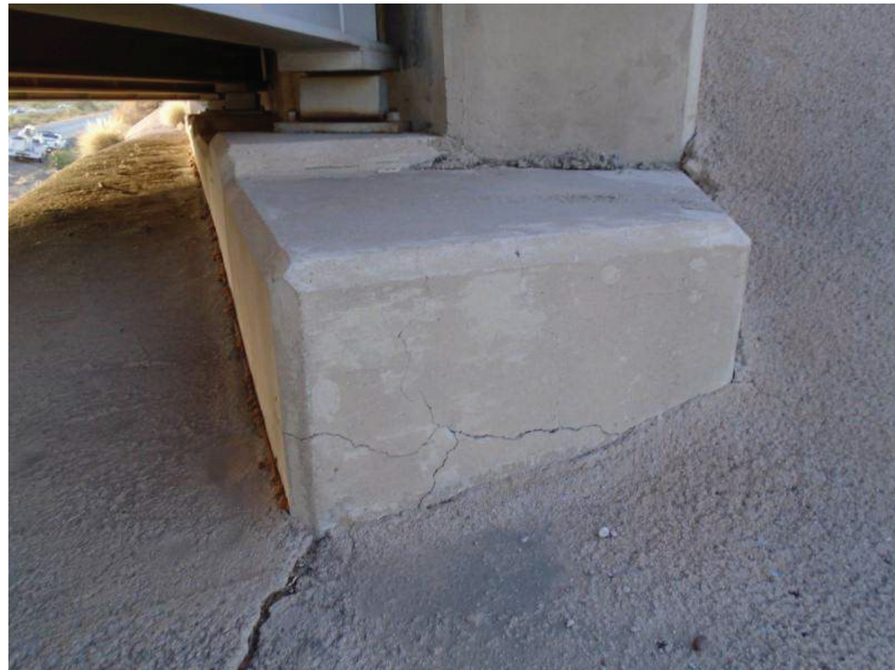
File Name : 01150-2020-05-31-Photo-19.JPG Description : Wide Map Cracks, East End of North Abutment, LNW
