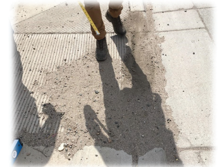
1383472 Curb Ramp Gravel on Ramp
