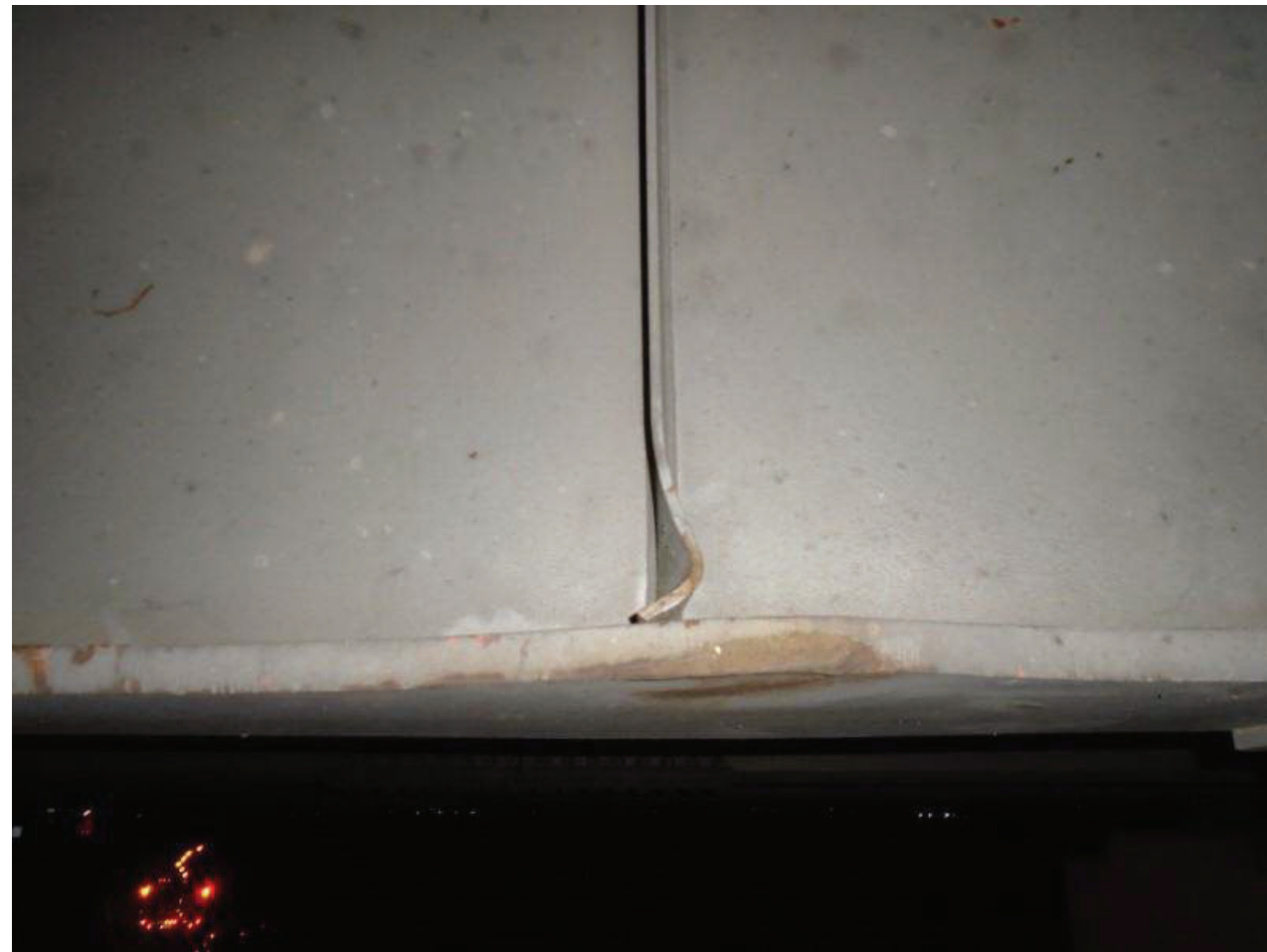
File Name : 01216-2020-05-31-Photo-23.JPG Description : Bent Vertical Stiffener, Span 2, Girder 2, Near East Splice Plate, LN
