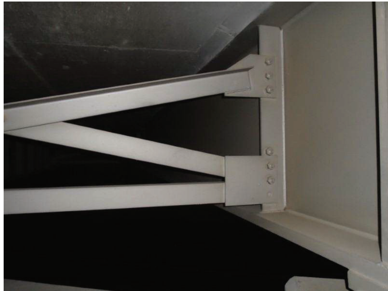
File Name : 01151-2020-05-22-Photo-18.JPG Description : Misaligned Diaphragm Bolt Hole, Girder 3, N Side of Pier 2, LS
