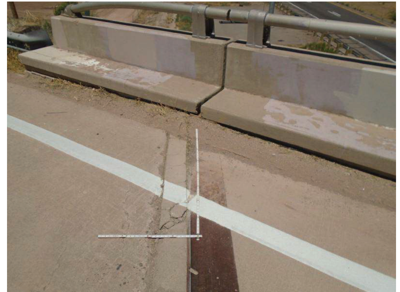
File Name : 01216-2020-05-31-Photo-10.JPG Description : Restricted Joint Movement, West Abutment Joint, LN
