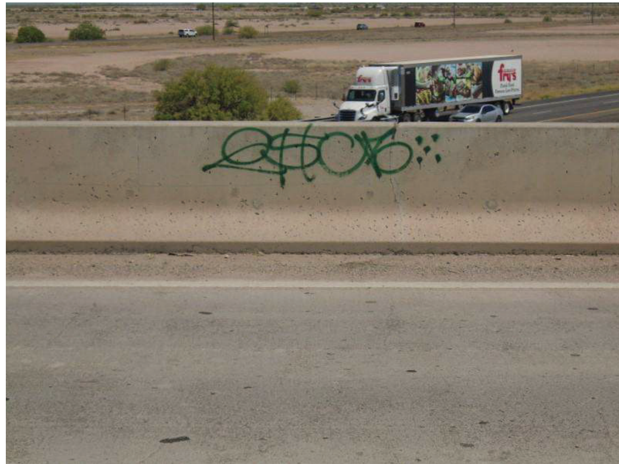
File Name : 01214-2020-05-31-Photo-10.JPG Description : Typical Graffiti, E Concrete Bridge Barrier, LSE
