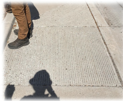
1383462 Curb Ramp No Truncated Domes
