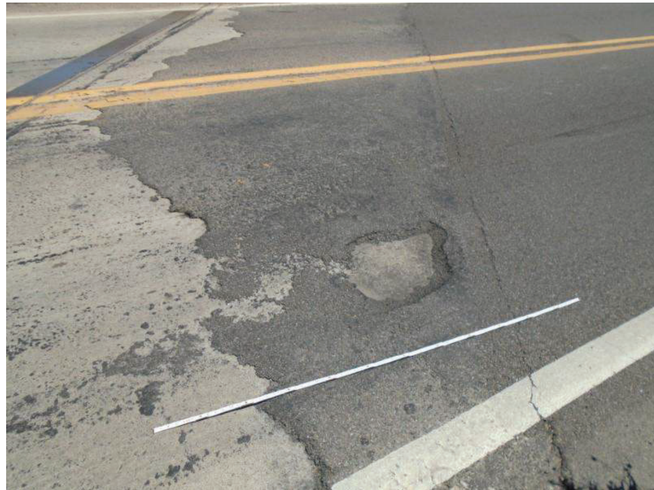
File Name : 01214-2020-05-31-Photo-8.JPG Description : Pothole, SW Approach Overlay, LSE
