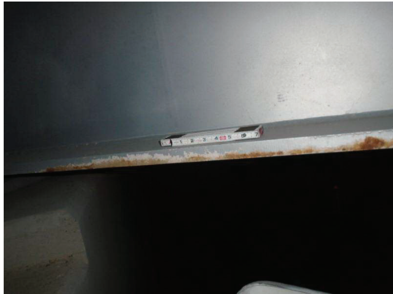
File Name : 01216-2020-05-31-Photo-29.JPG Description : Failing Paint, Span 3, Girder 1, Near Pier 3, LN
