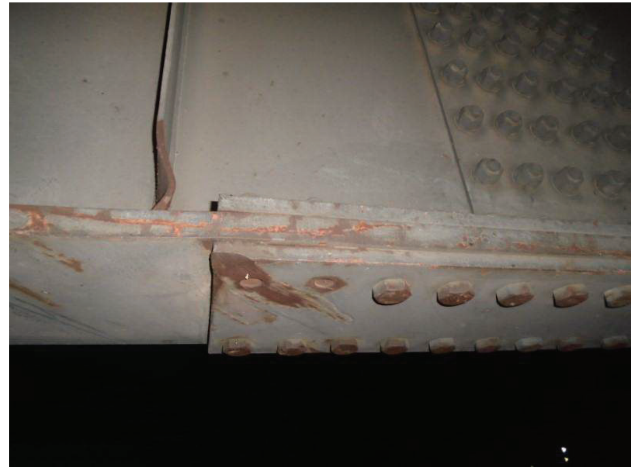
File Name : 01214-2020-05-31-Photo-21.JPG Description : Sheared Bolts, Span 3, Girder 1, South Splice Plate, LE
