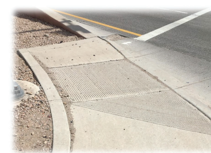
1383474 Curb Ramp No Truncated Domes
