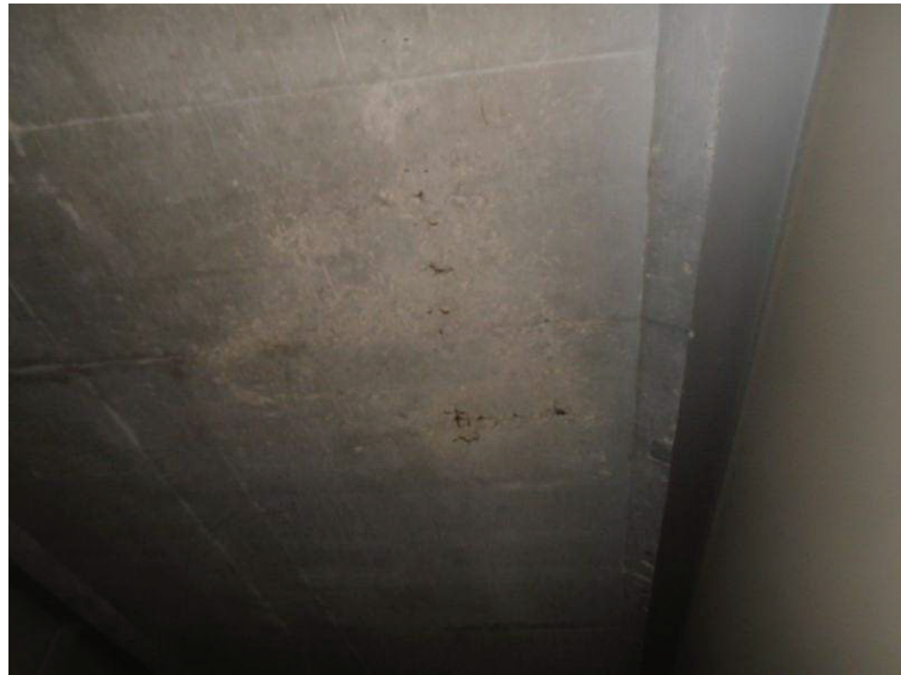
File Name : 01214-2020-05-31-Photo-28.JPG Description : Soffit Honeycombing with Exposed Rebar, Span 2, Bay 3
