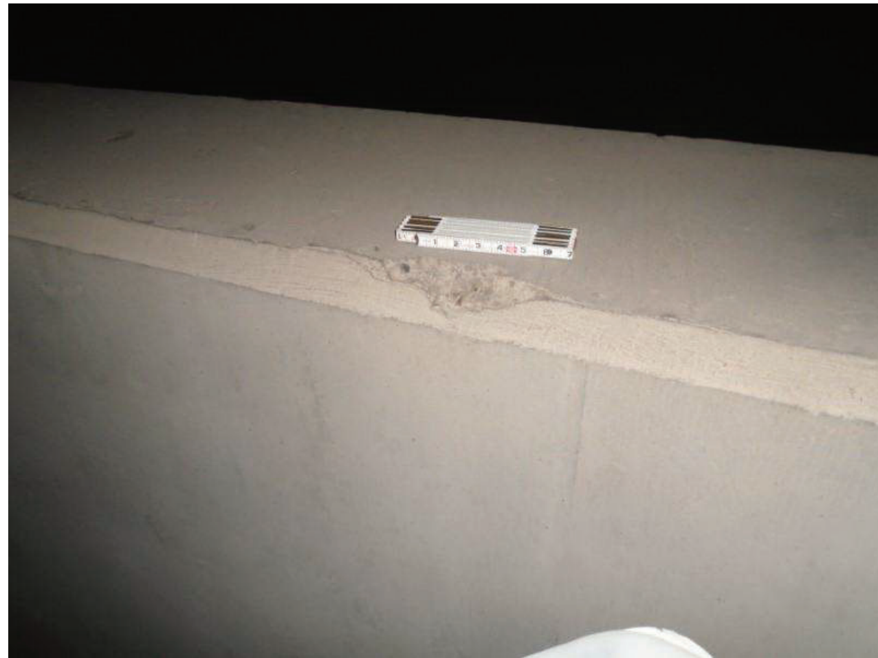
File Name : 01214-2020-05-31-Photo-26.JPG Description : Edge Spall, Pier 1 Cap, Bay 2, South Side, LN
