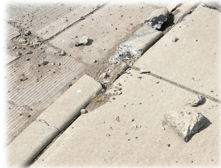
1028011 Sidwalk Broken Concrete
