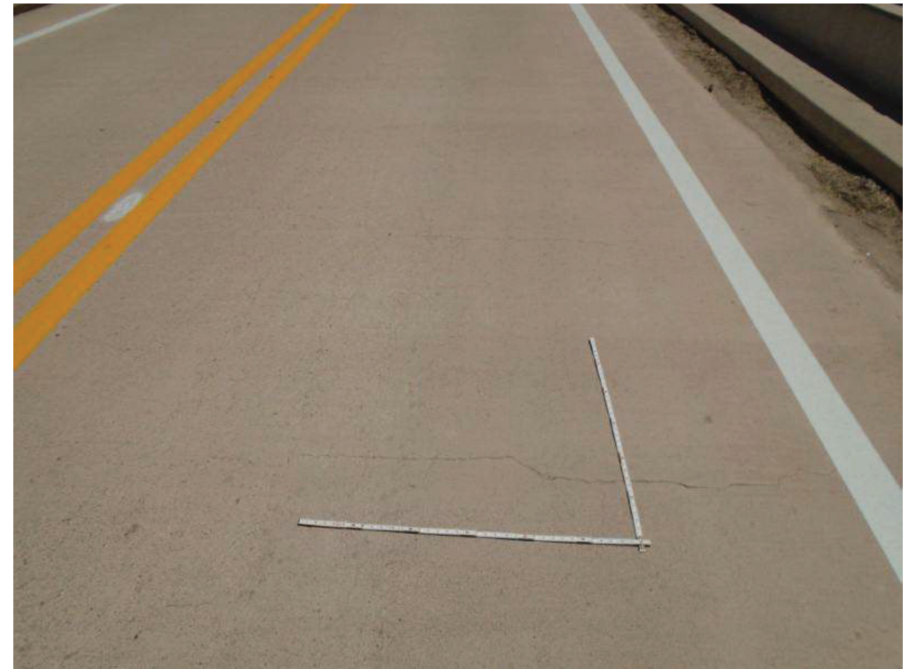
File Name : 01216-2020-05-31-Photo-6.JPG Description : Typical Deck Cracking
