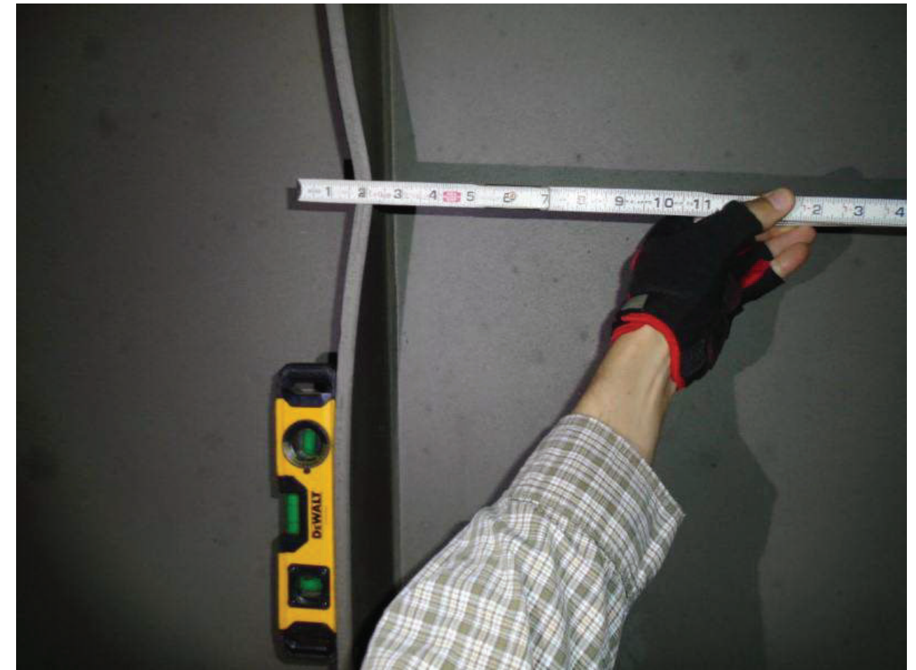
File Name : 01151-2020-05-22-Photo-19.JPG Description : Bent Stiffener, 7th From Pier 1, LE
