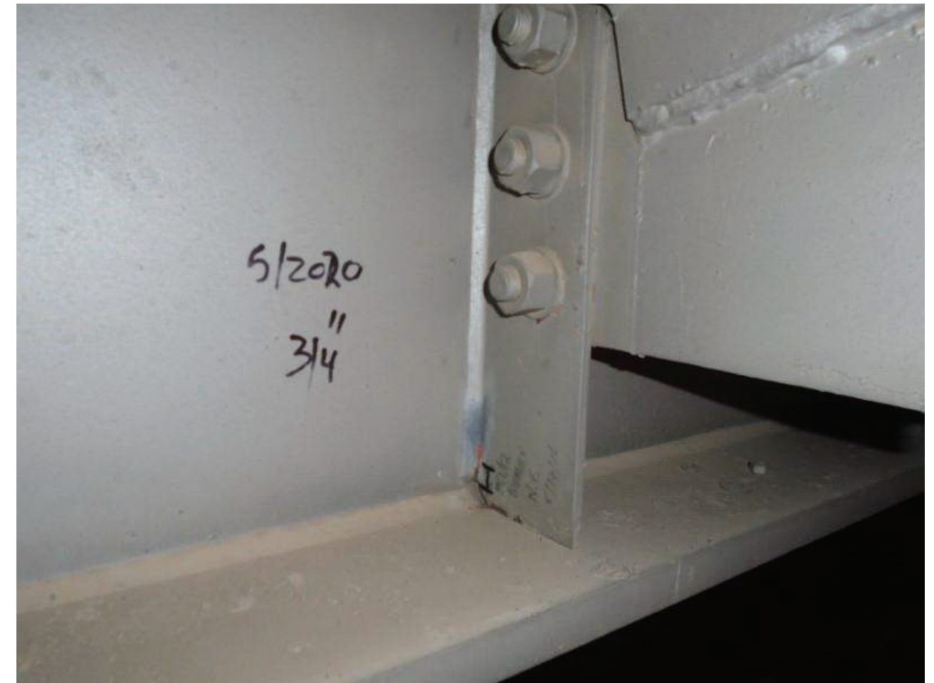
File Name : 01216-2020-05-31-Photo-28.JPG Description : Crack in Vertical Stiffener, Span 2, Girder 1, Diaphragm 2, LS
