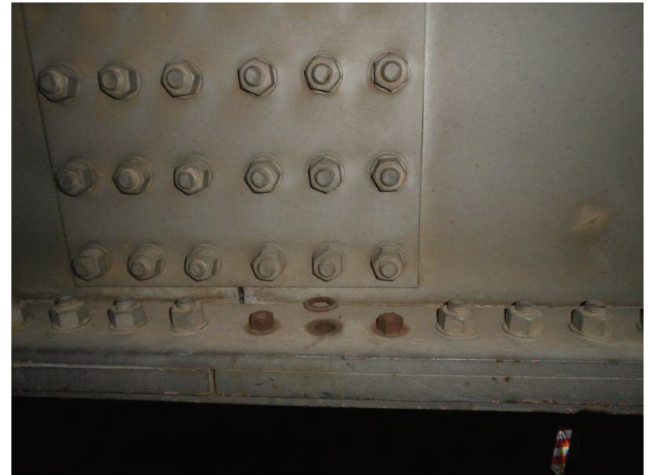
File Name : 01215-2020-05-31-Photo-25.JPG Description : Missing Bolt, Span 2, Girder 4, South Splice Plate, LE
