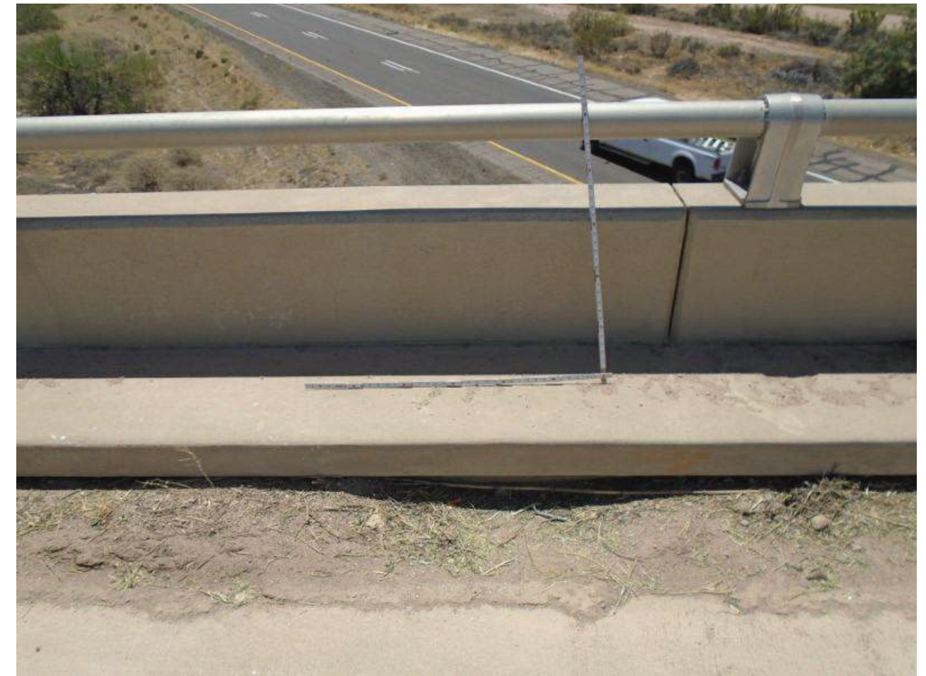
File Name : 01216-2020-05-31-Photo-12.JPG Description : Typical Shoulder Debris, Both Sides of Bridge
