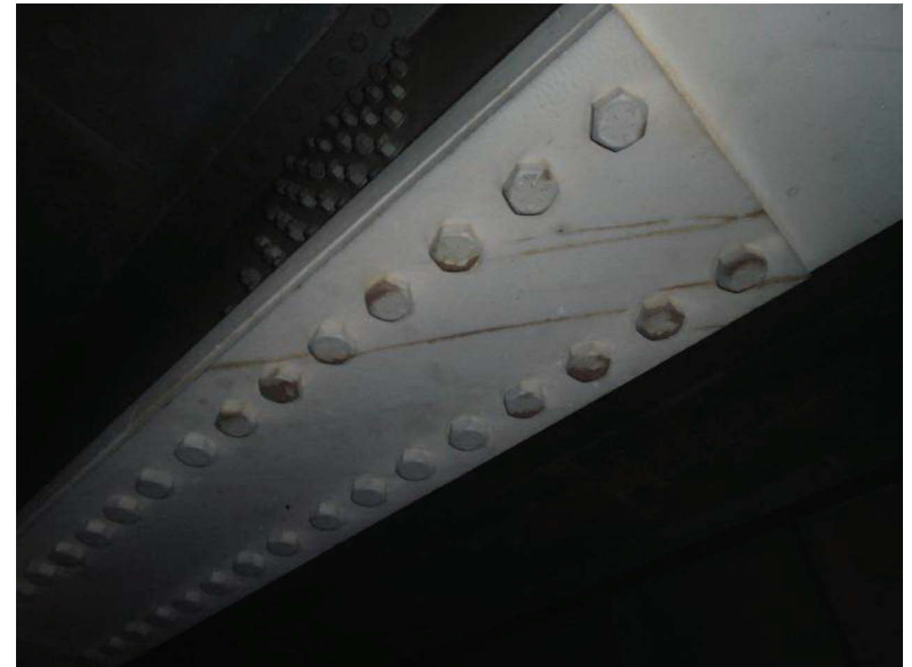
File Name : 01215-2020-05-31-Photo-19.JPG Description : Scrape Marks, Bottom Flange, Girder 2, Span 4, Under N Splice Plate
