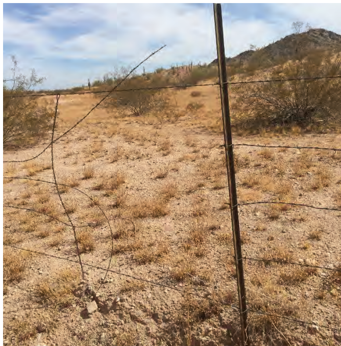
Figure 1. Damage to fencing along I-10.
