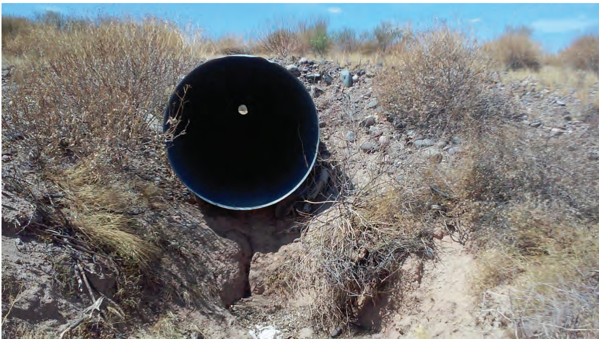
Figure 4. Culvert with natural substrate eroded.
