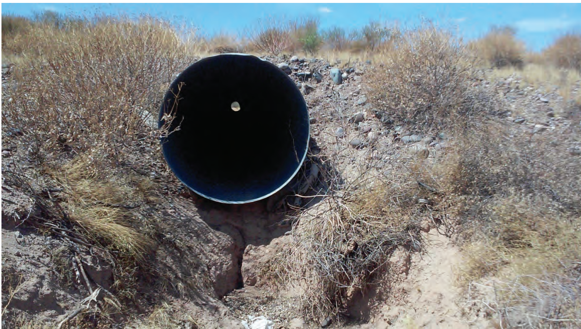
Figure 4. Culvert with natural substrate eroded.
