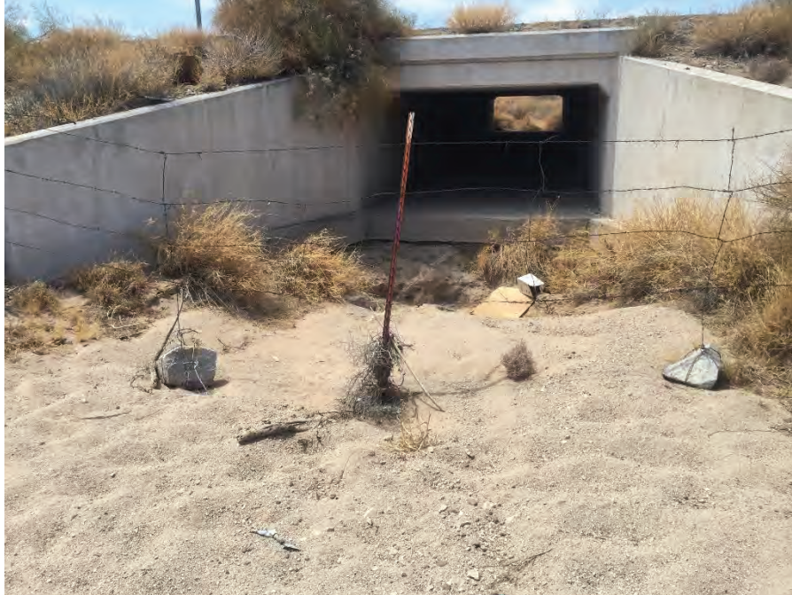
Figure 2. Erosion along fencing allowing terrestrial wildlife to enter the I-10 ROW.
